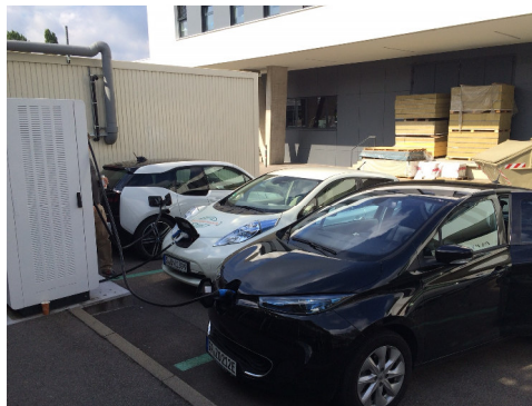
Picture 3: Installation of one of the first Multi-Chargers with 150kW at the Fraunhofer IAO, Nobelstr., Stuttgart, 2016
