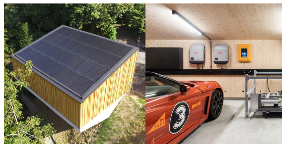
Figure 7: S2W Pilot Installation in Switzerland. On the left it is possible to see the second-life battery and, on the wall, the inverters and the controller
