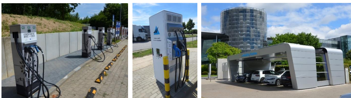
Figure 6: Examples of recently installed fast-charging infrastructure (Autobahn A14 near Nossen; Autobahn A4 near Bautzen; at “The Transparent Factory” of Volkswagen in Dresden (including solar panels and storage))
