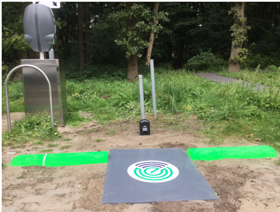
Figure 3: The wireless charging station in Rotterdam
