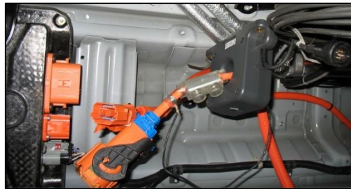
Figure 4: Picture of the disconnected high-voltage battery main cable, modified to include a 2AWG cable with a high current fuse through which a 500A solid-core amp probe is looped
