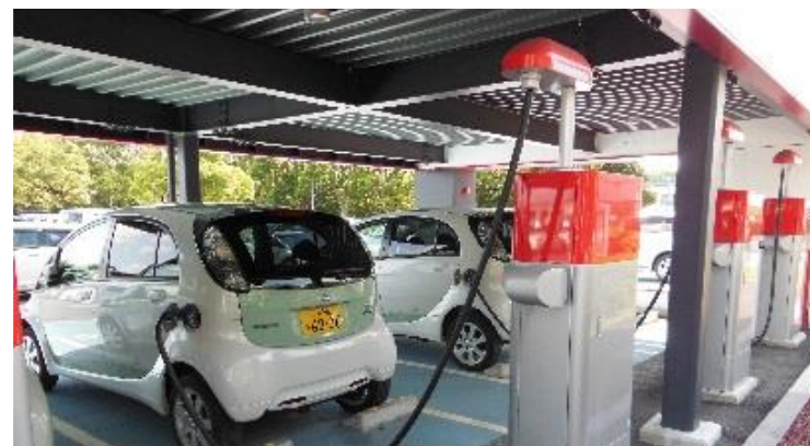
Workplace charging and application to V2X at Mitsubishi
