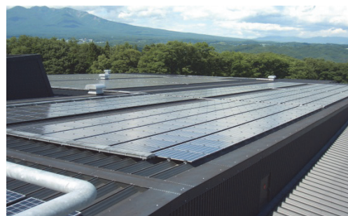
Figure11: 490kW PV System
