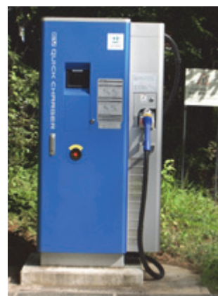
Figure4: CHAdeMO (Rapid Charging System)
